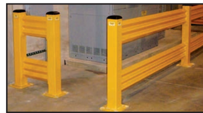
Guarding Electrical Panels
