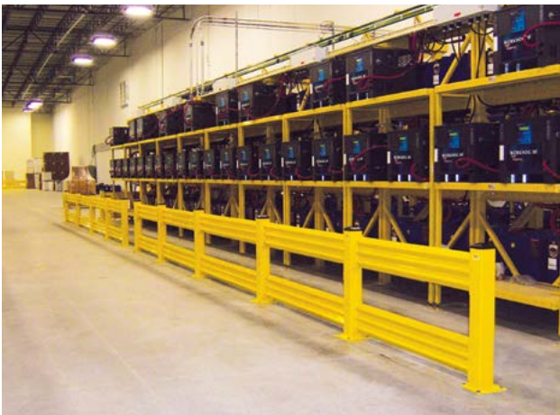
Guarding battery racks
